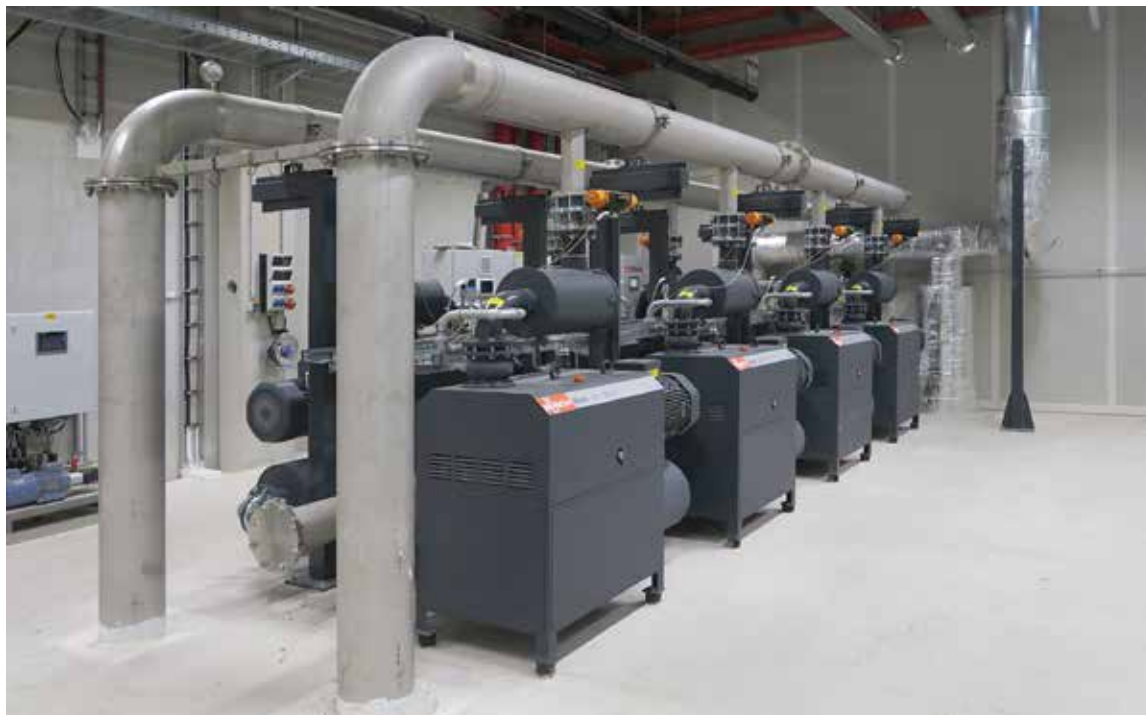
Left: Busch's central vacuum system with Mink claw vacuum pumps.
